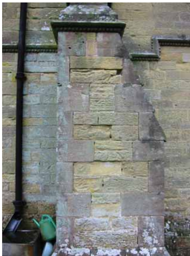
Figure 36. Yellow Farlow Sandstone in the centre of this buttress for the nave of the church, Cleeton St Mary. Quoins are of red-brown Felton Stone.
