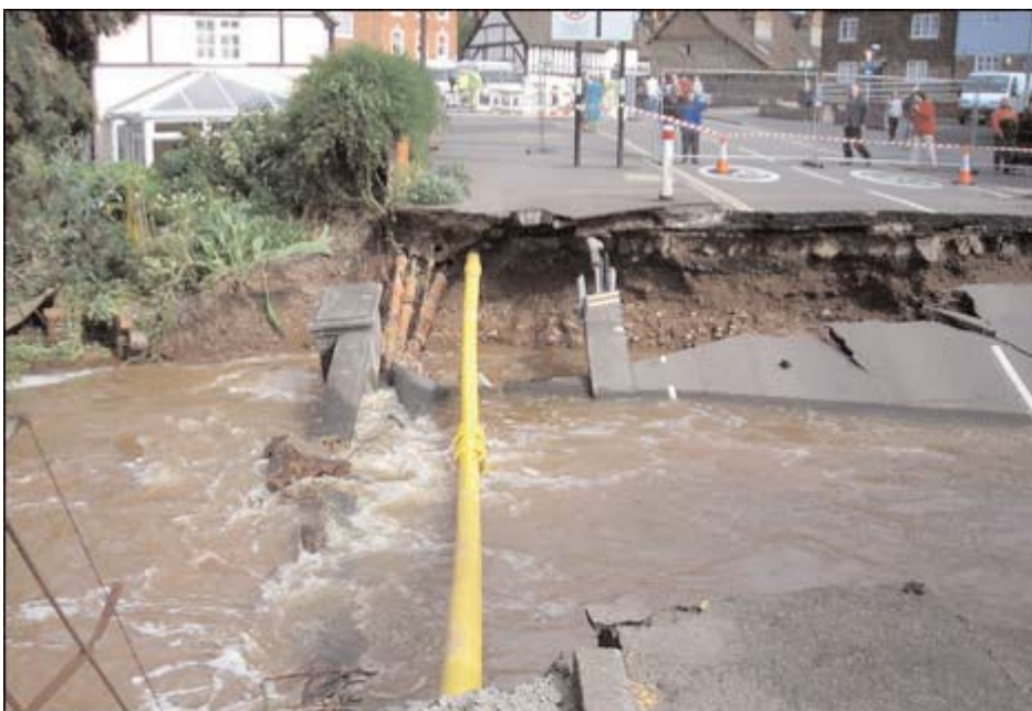
The collapsed Burway Bridge; until Monday 25th June 2007 this carried the former A49 (Coronation Avenue) over the River Corve south into the centre of Ludlow.
